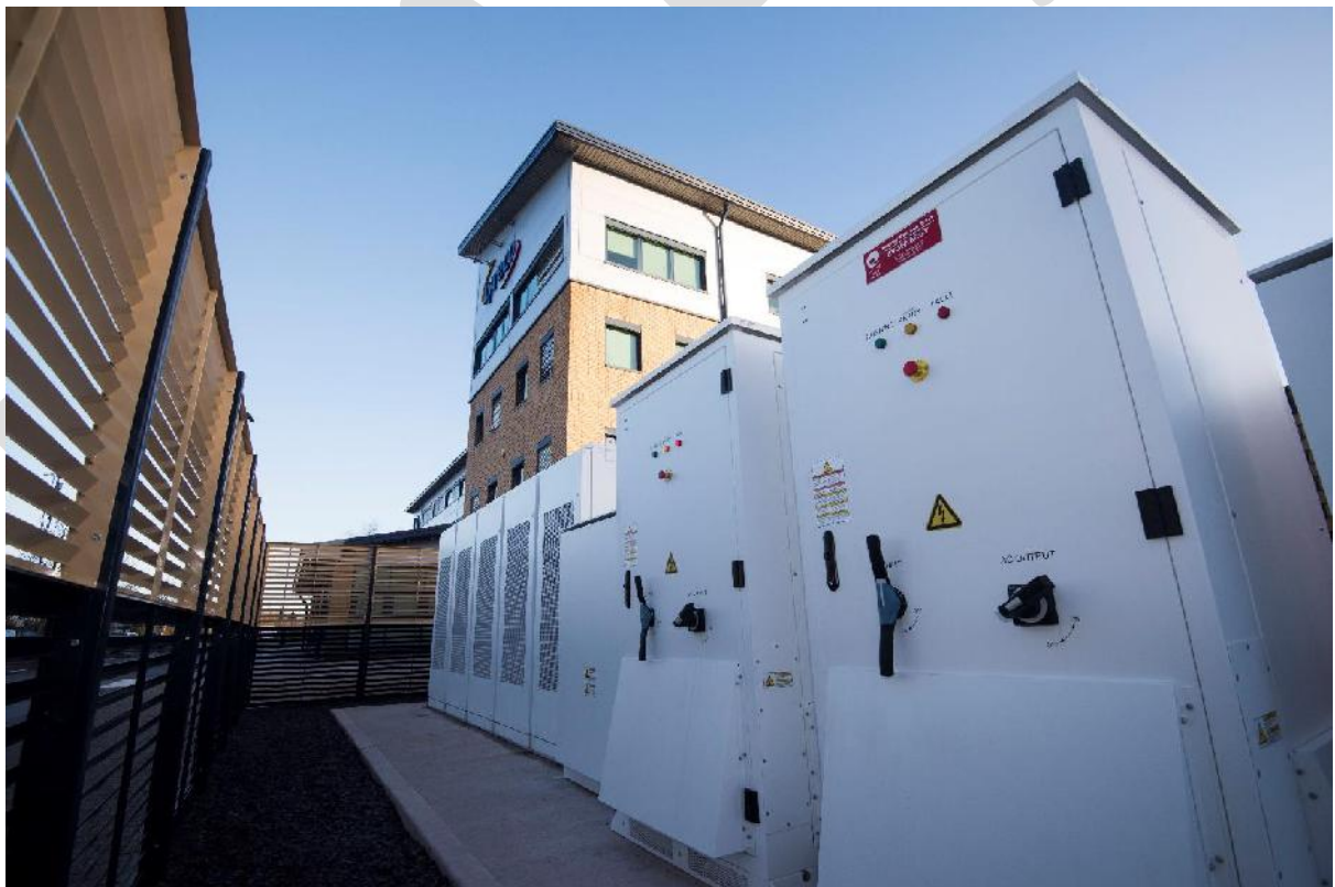
Figure 8: Example battery storage facility
